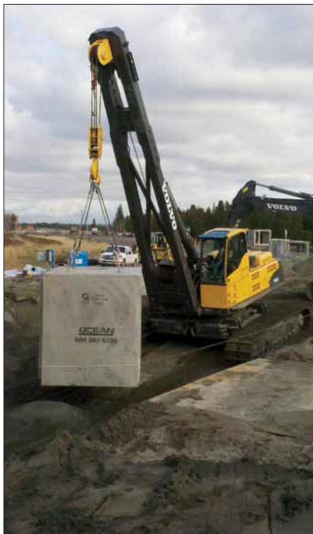
Brother Oliver Cordts installing box culvert sections with a Volvo PL4611 pipe layer for Greenbelt Excavating on the South Fraser Perimeter Road. Photo by Brother Al Cooper.
