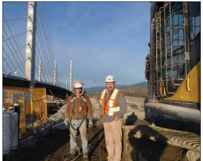
Brother Shawn MacLeod and a member of Local 1611 assisting in the demolition of the Pitt River Bridge for Pacific Blasting.
