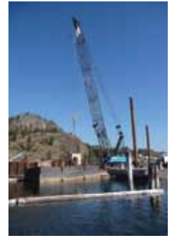
COVER PHOTO—Brother Dave Zimmer dismantling the graving docks during the construction of the Kelowna Bridge. —Photo by Tricia Borys
